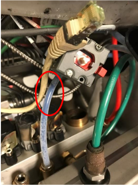
Soot inside the air hose
